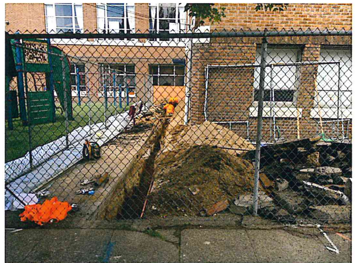
Copper pipes are placed along the southwest edge of School Building
