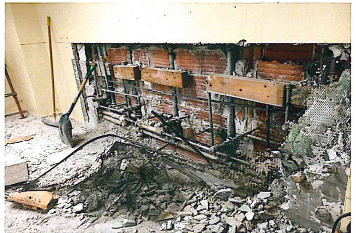
Old pipes are exposed in the Boys Restroom
